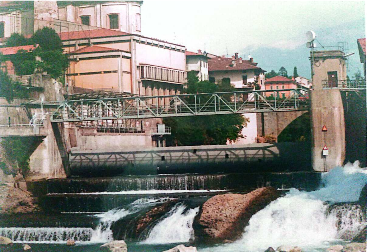
Artificial barrier located in Ponte San Pietro which prevent the upstream movements of aquatic animals into the Brembo River Zone (WGS84 coordinates: 45°41'45.4"N 9°35'25.2"E)
