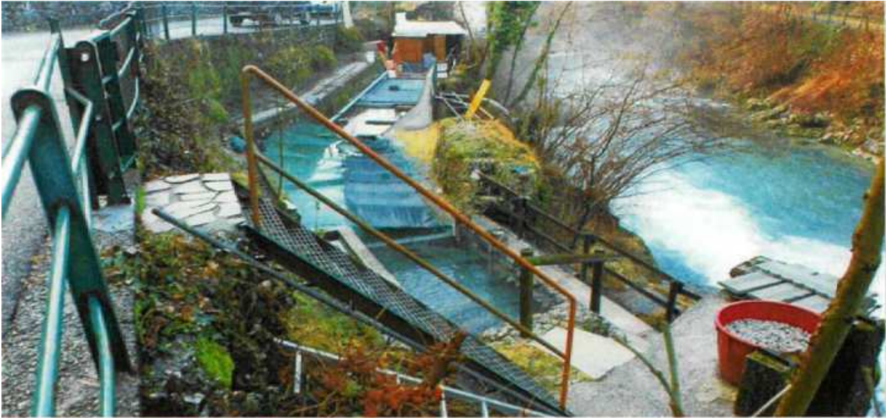
View of the establishment in the municipality of Ponte Nossana, in Località Sorgenti, near to the Nossana torrent
