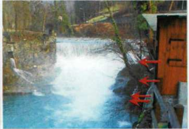
Side view of the structure. On the wall, some of the outlets discharging waters in the Nossana torrent are visible
