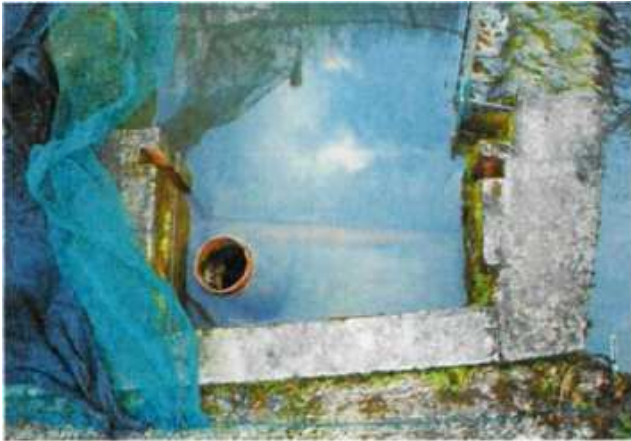
Detail of one of the drains of the external concrete tanks with level regulation pipes and guides for the protection grid
